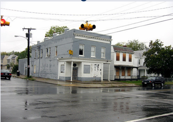
Renovations are underway for a new "99¢" store at the corner of Fairmount and North 22 nd Streets.
